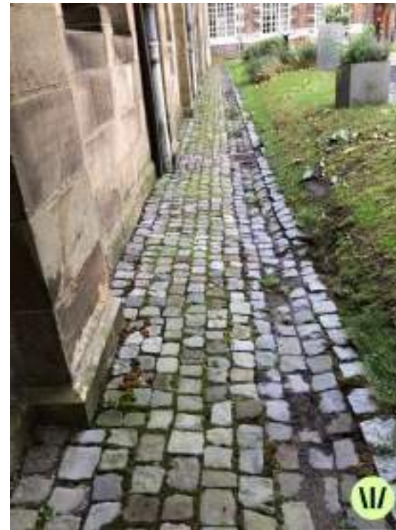
Gutter too deep
